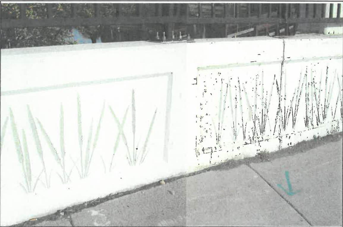
Picture 4: Painted (left side) compared to Unpainted (right side)
